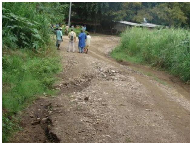
Illustration 4.2.: gully crossing the road
